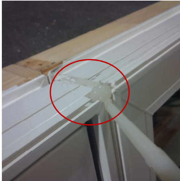
Figure 1: Silicone sealant applied across exterior edge of product, and corner cleaned area.
